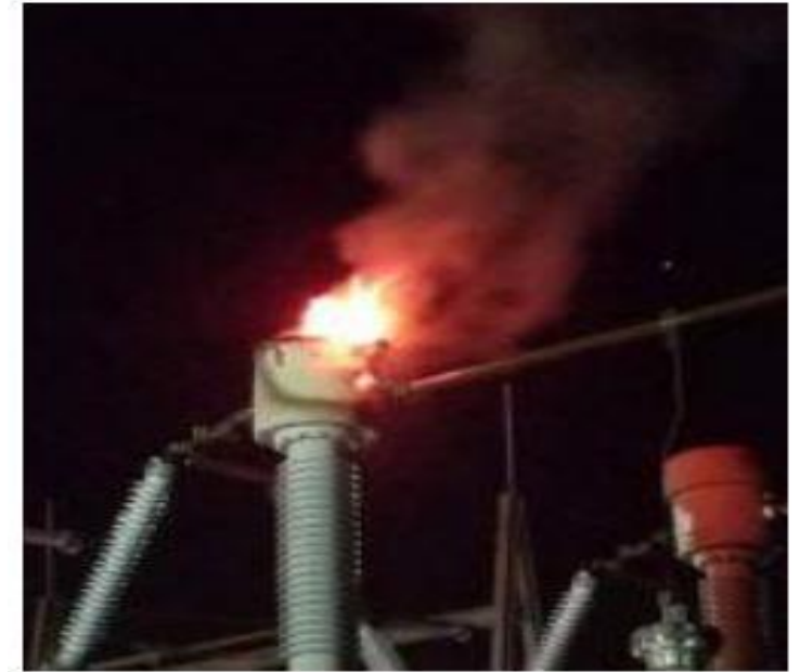
Figure 2: C-phase CT failure [1]
