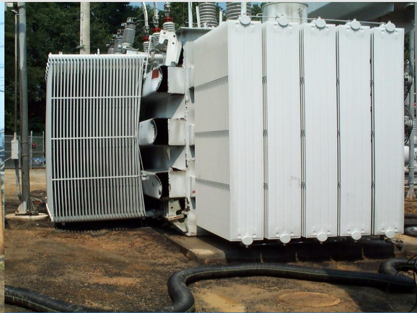
230 kV Transformer Failure in 2001
