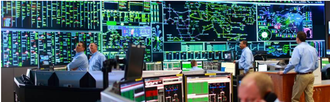
Figure 6. System Operations – PJM Control Room
